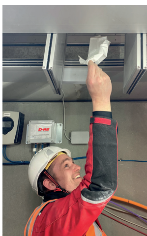
The handkerchief indicates the air flow in the shaft which carries valuable energy to the outside while the flap remains permanently open.
